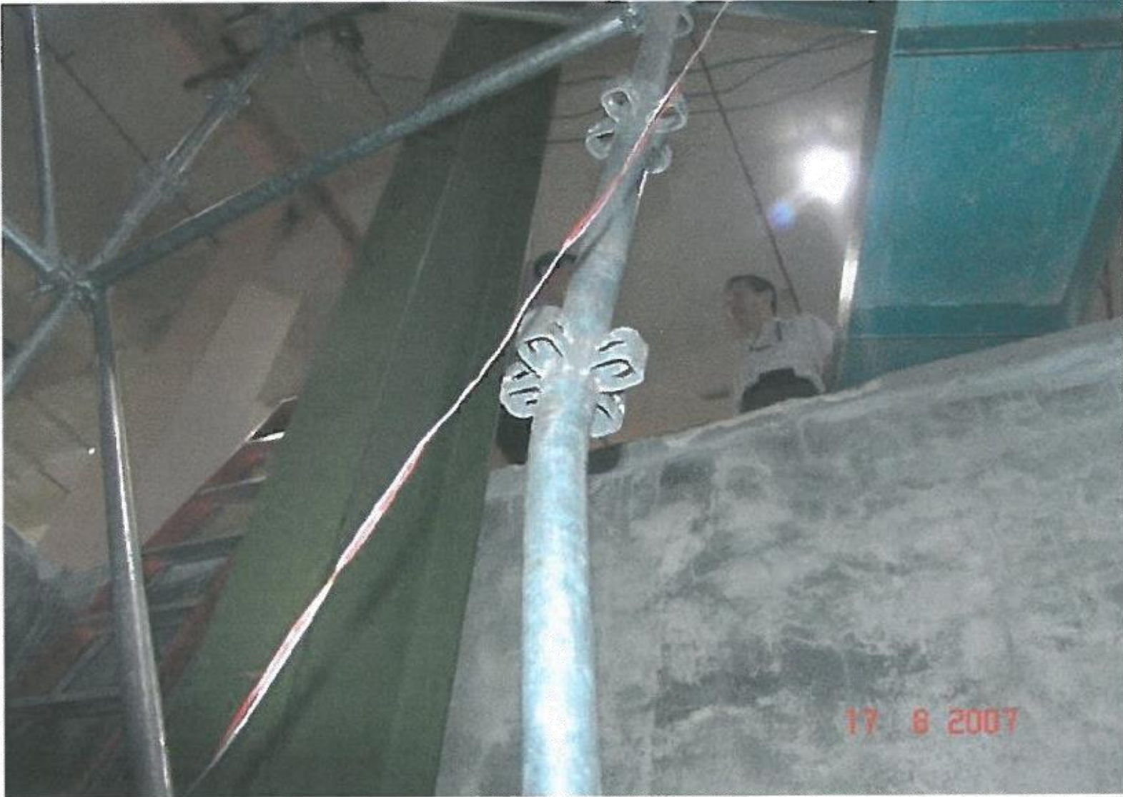
Picture 02: Buckling on the tower leg.
